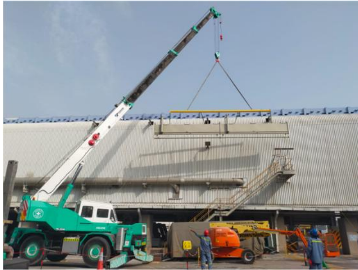
Figure 9. Lifting of horizontal distribution and transport air slide.
