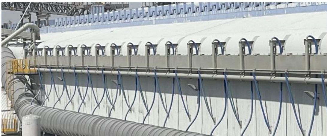
Figure 10. Installed alumina distribution and transport system.
