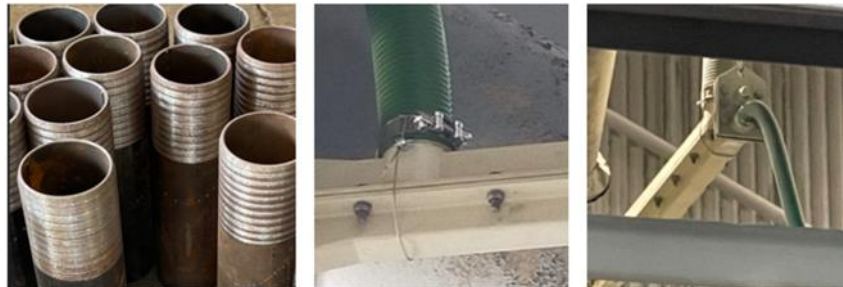
Figure 2. Serrated hose connections and securing wires for flexibles.
